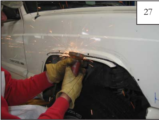
Use a cut off saw to cut the front fender along marked line. Do not cut any sheet metal past where the horizontal lines were marked in step 24. See next photo for fender image after trimming.
