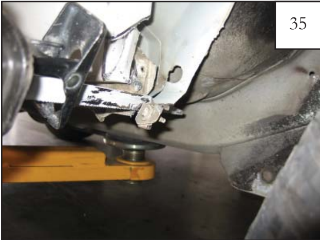
Use a saws all to cut off remaining sheet metal and bolt.
