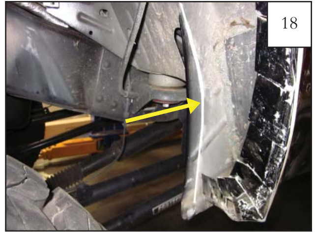
Draw a line along the inner wheel well wall that parallels the outer edge.
