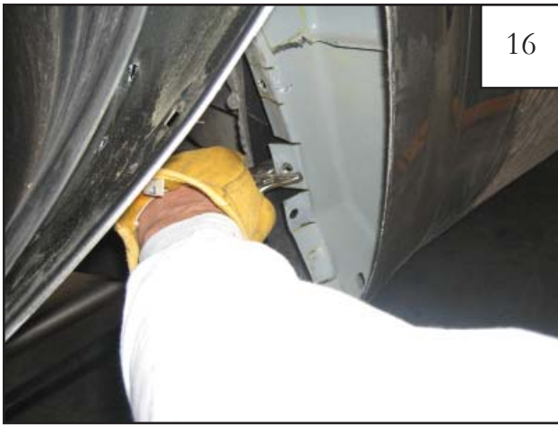
16 Bend lip straight with pliers between cuts made in previous step. NOTE: In Step 20, existing cuts will be extended after reference lines are marked.
